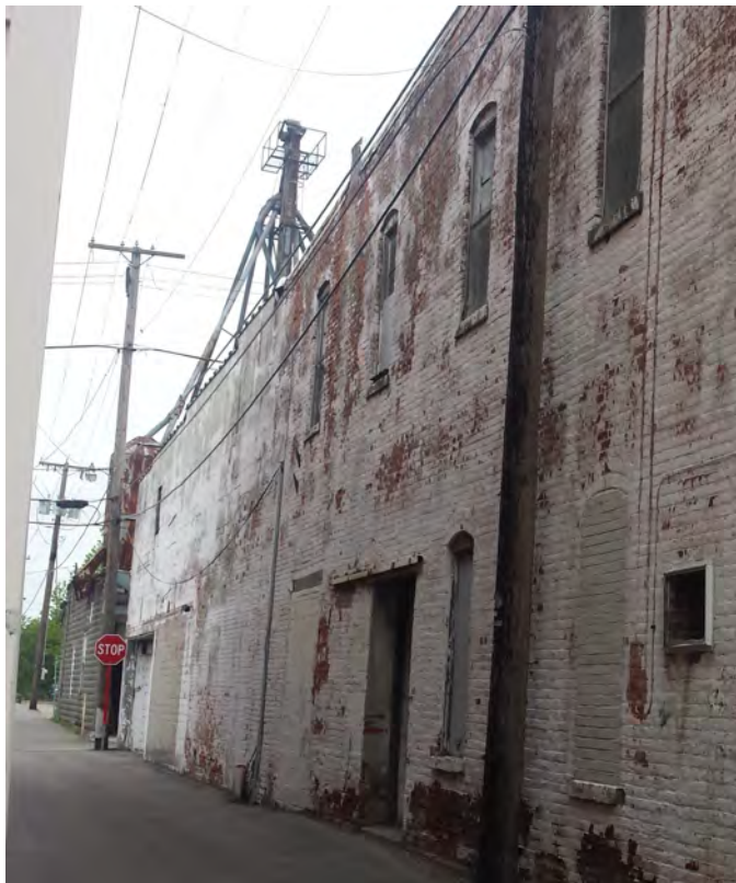
North elevation has similar issues as noted for the front elevation.
