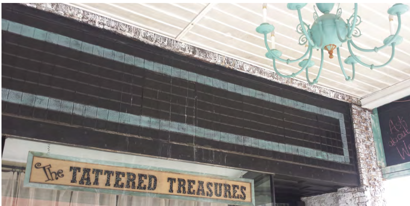
Transom detail. Paint from brick should be removed.
