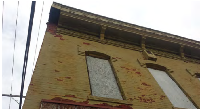
Painted brick is peeling, and windows are boarded up.
