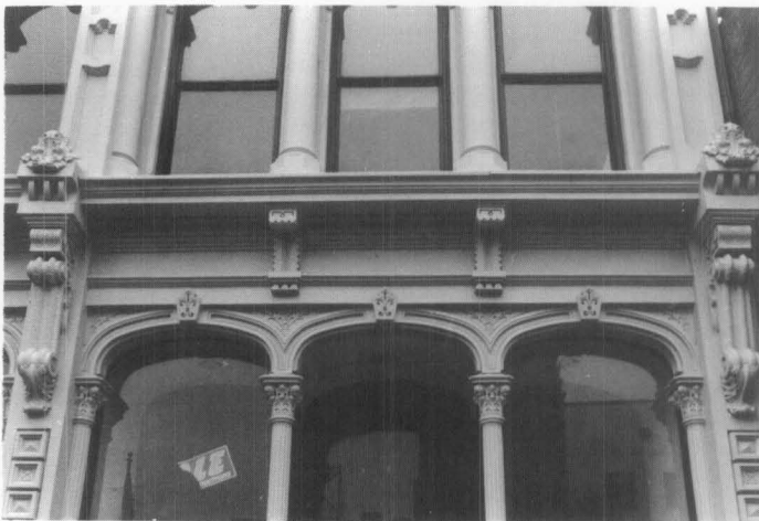
Figure 8. When the Grand Opera House in Wilmington, Delaware, was rehabilitated, missing cast-iron columns were cast of aluminum to match the original; in this particular case, because these columns do not carry great loads, aluminum proved to be successful substitute. Photo: John G. Waite
