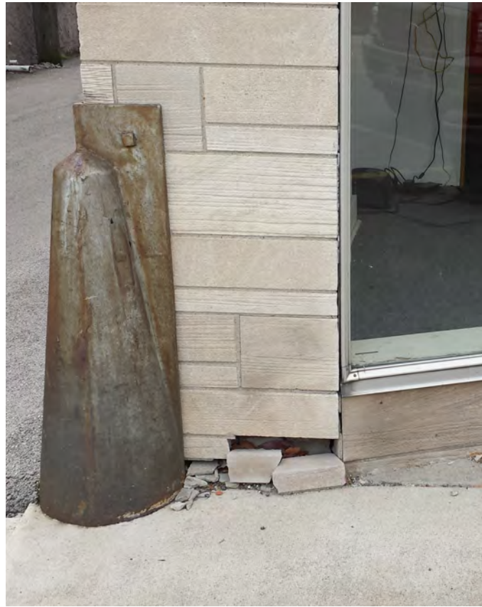
The limestone façade requires minor repairs, although ideally, it should be removed to bring it back to its original Italianate-style appearance. The image below shows the north wall with attractive brick design, but infilled windows and door. Tuckpointing is needed.
