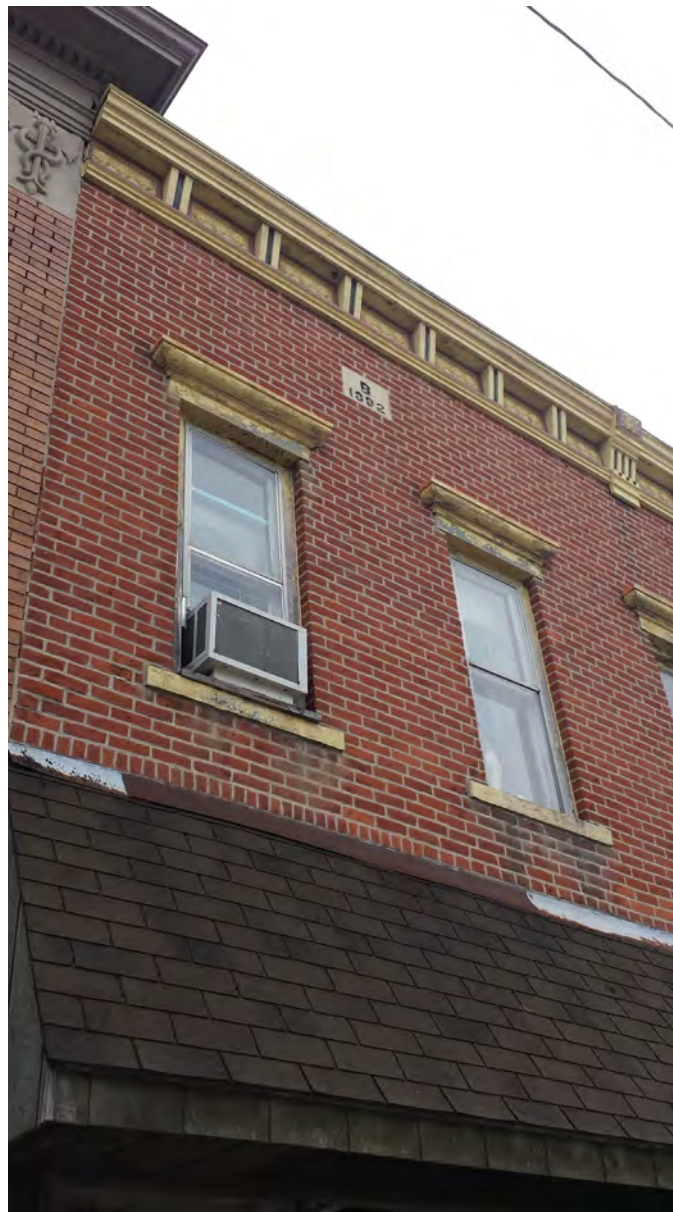
The cornice, window head, and window sills appear to be the original ornamentation and should be maintained.
