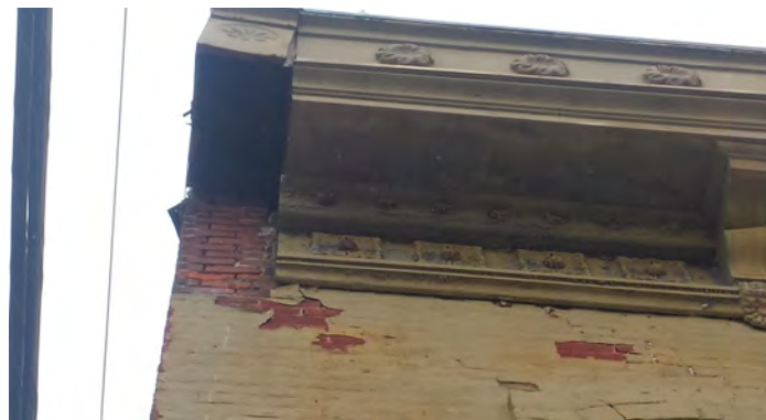
Cornice segment needs replacing, and tuckpointing is needed.
