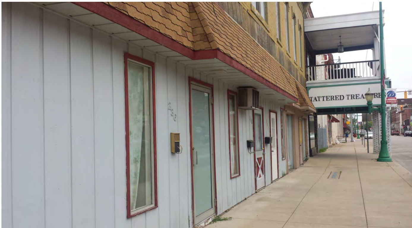
Wood siding, asphalt shingled awning, and inappropriate doors and windows should be removed.
